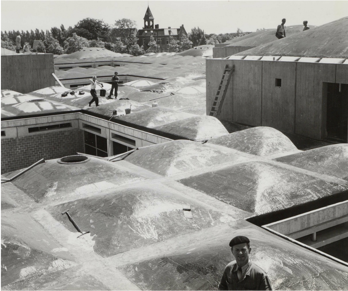
Amsterdam Civic Orphanage IJsbaanpad (arch. Aldo van Eijck) during construction 1959, Stadsarchief Amsterdam / J.W. Arsath Ro'is
